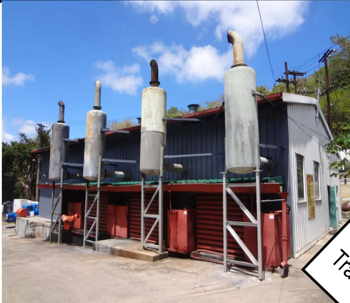
Diesel Generator Power Plant in Bequia
