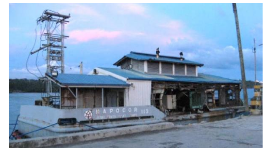
Mobile diesel generation unit – Siquijor Island, Philippines (Bertheau, 2013).
