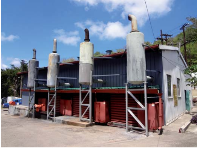
Figure 2.2: Picture of diesel power plant on the island Bequia, St. Vincent and the Grenadines, own photo source
