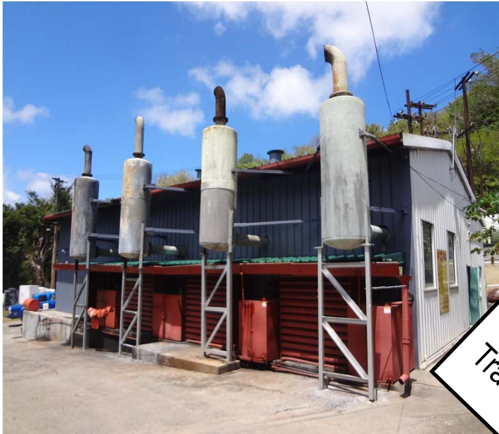
Diesel power plant in Bequia
