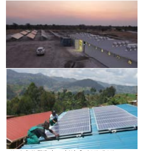
photos: top: Namibia, 2010; left: solar power plant, below: Rwanda, training of technicians © 2014 SMA Group
